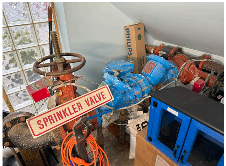
Fire Sprinkler Service
