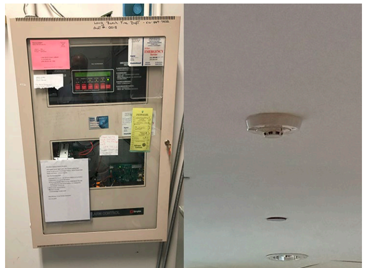
Fire Alarm System
