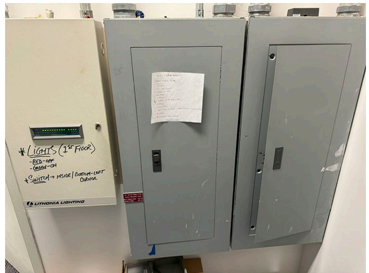
Power & Lighting Panels
