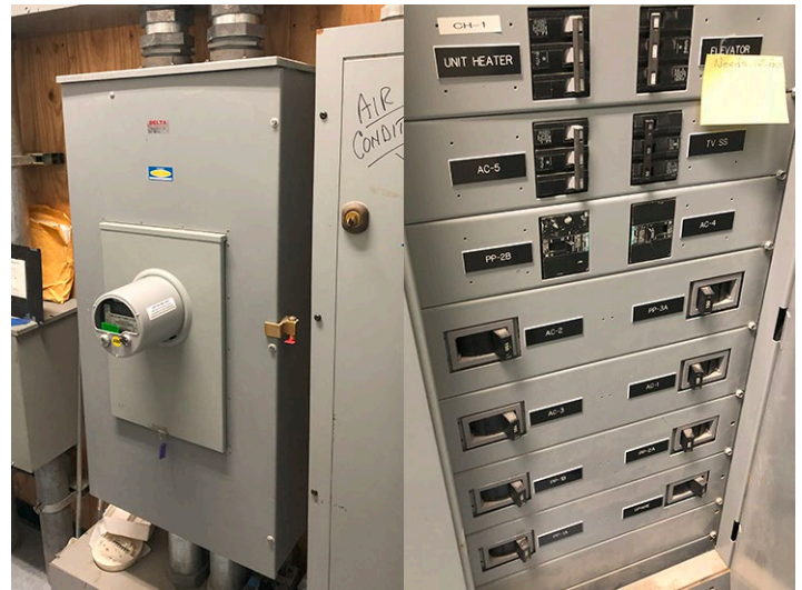
Electrical Service Entrance & Main Distribution Panel
