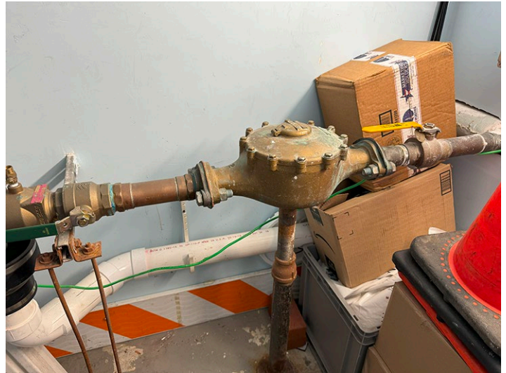
Water Service & Hot Water Heater
