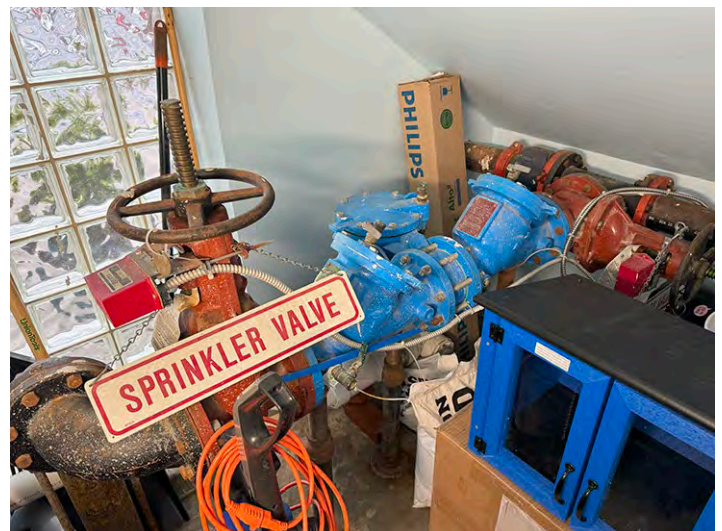
Fire Sprinkler Service
