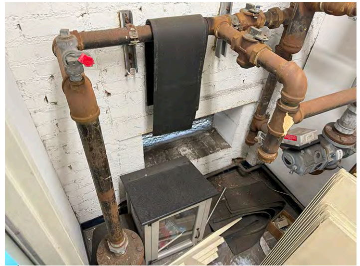
Natural Gas Service
