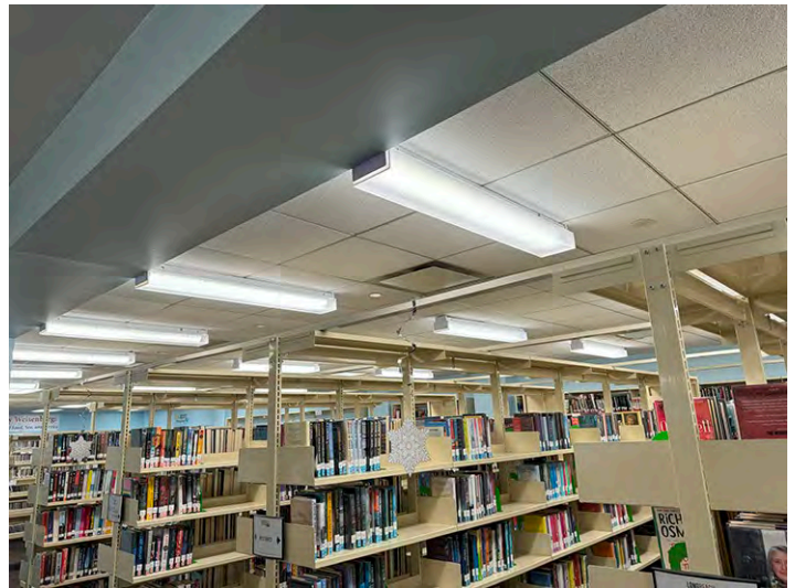
Main Level Lighting
