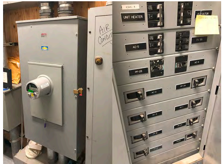
Electrical Service Entrance & Main Distribution Panel
