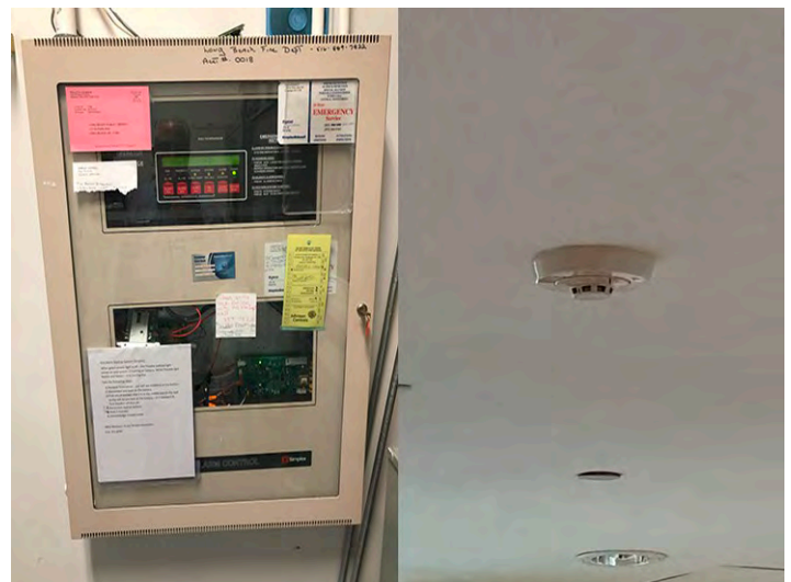
Fire Alarm System
