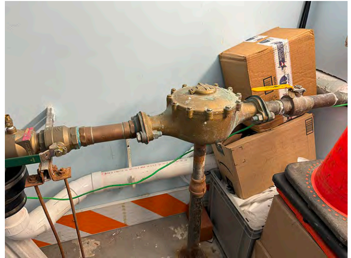
Water Service & Hot Water Heater
