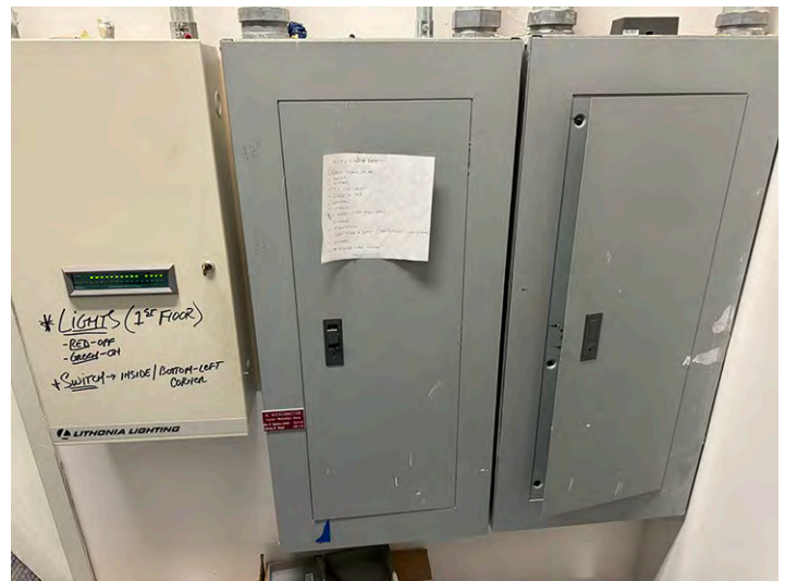
Power & Lighting Panels
