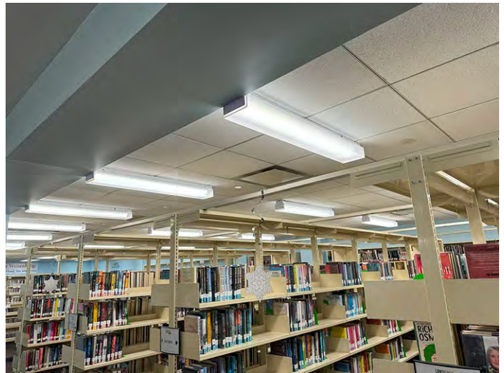
Main Level Lighting
