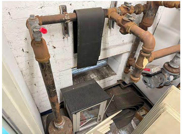
Natural Gas Service
