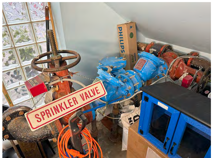
Fire Sprinkler Service
