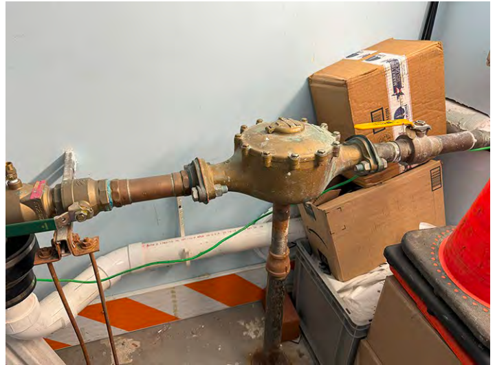
Water Service & Hot Water Heater
