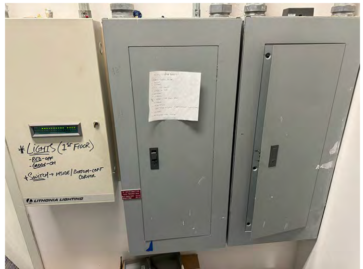
Power & Lighting Panels
