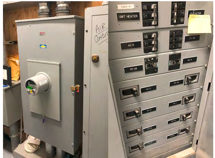
Electrical Service Entrance & Main Distribution Panel
