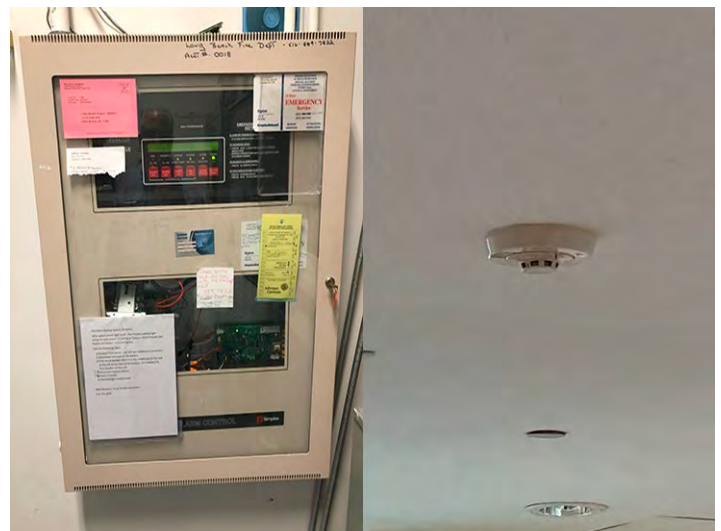
Fire Alarm System
